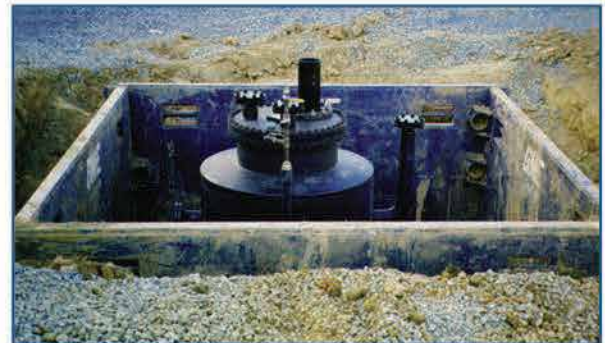
GME shields in a pit application.
